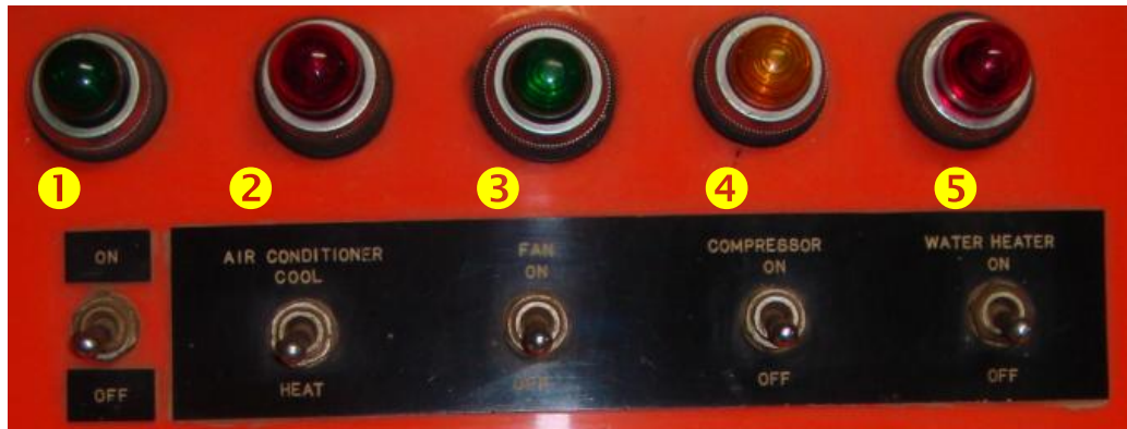
Figure 4 Main control panel
