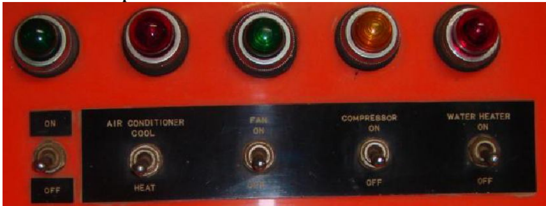
Figure 4 Main control panel
