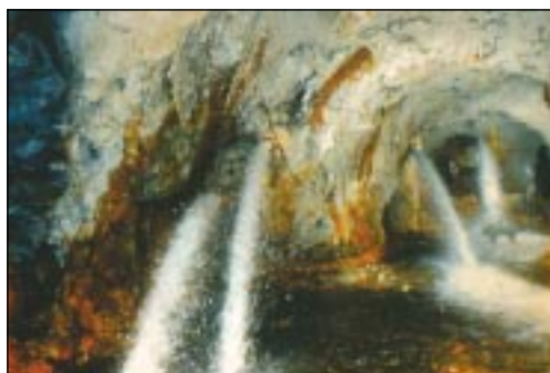
Photo 8 – Water flow into Saint Guillaume II tunnel from Grange Pellorce fault, France
